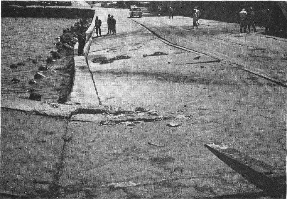
Photo. 14 Subsided Wharf in Aomori City
