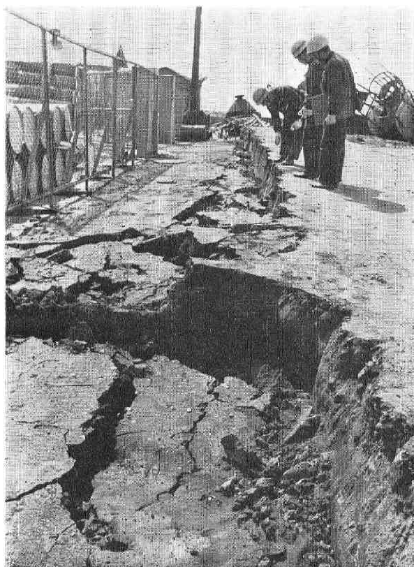
Photo. 12 Fissured yard, Mitsubishi Petroleum Co., Hakodate City
