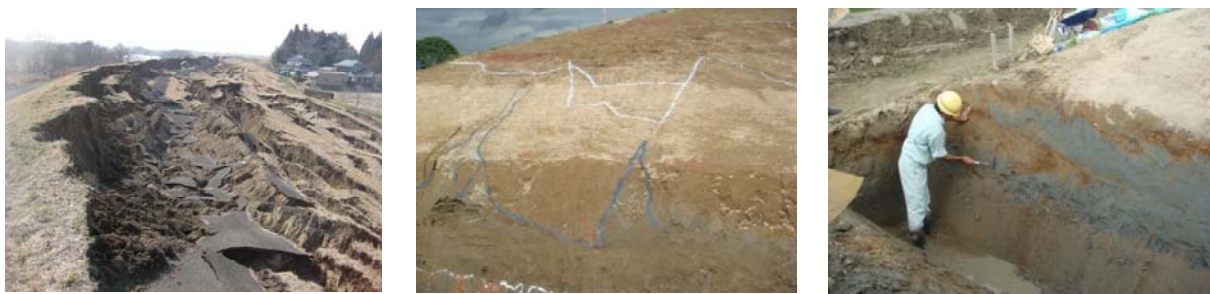
Fig. 6 (left) the disaster area (the inside of the dike is shown on the left side, seen from downstream to upstream) (center) liquefaction trace verified by the open cut investigation (marker points indicate the trace of liquefied sand which penetrates into the inside of the dike) (right) cross-section of the open cut investigation : trace of squeeze of liquefied sand was confirmed
