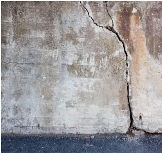
c) crack in wall ( do not consider)
