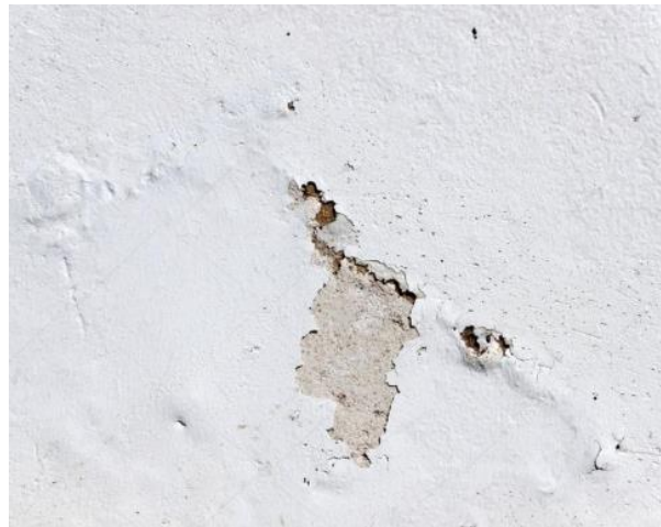
d) plaster deterioration ( do not consider)
