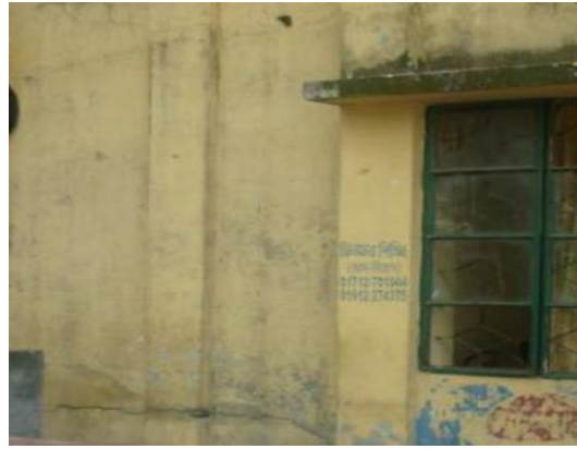
(b) Crack through RC column ( consider)
