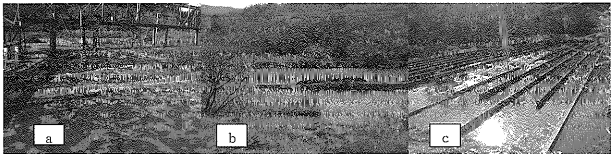
Fig.1. Operation unit of swine wastewater treatment plant. a: SBR, b: oxyc pool, c: baffle channel.
