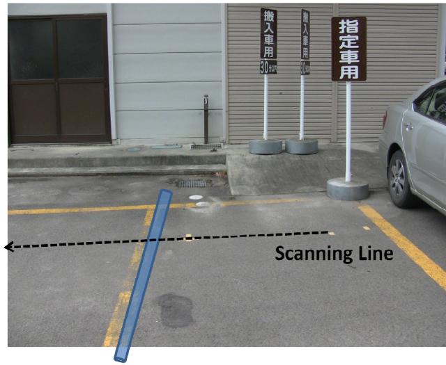
Fig. 4.2. GPR experiment configuration for a buried pipe detection. The scanning line is shown with an arrow line
